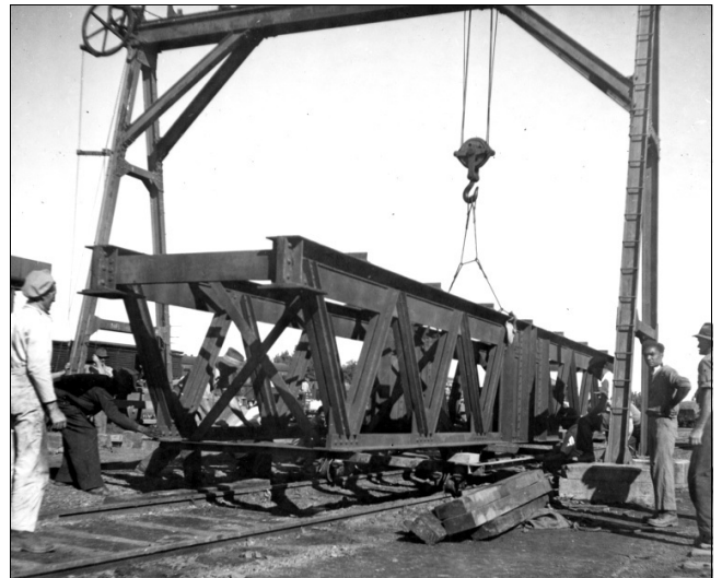
Once the load was taken by the crane the jinker was moved away and the span lowered onto railway wheels or track rollers.
