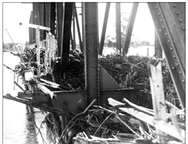
The remnants of the pedestrian walkway on the west side of the bridge, immediately after the flood. Source: NSW Railways Photo ARHS 126892
