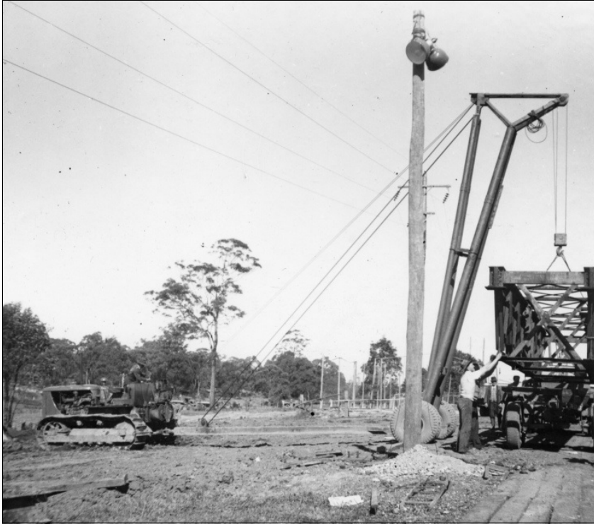
Transferring a Warren truss span from rail to road at Middleton Street level crossing. Note the arrangement of the crane with caterpillar tractor, the beam to the rubber-tyred axle and the shear leg tied back to the tractor.
