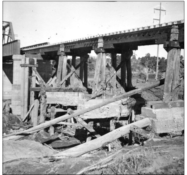
The 1949 repairs to the No.1 viaduct section, as exposed in 1950 and seen from the east (downstream) side of the bridge. Originally the structure would have been simply driven timber piles, but the concrete pile caps were added after flood damage and 35 years of rot at ground level. Source: NSW Railways Photo ARHS 126879.
