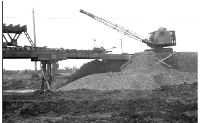
While the No.3 viaduct section was largely undamaged, its Sydney-end abutment was destroyed. Here a dragline makes repairs, while to the left, wrought iron Warren trusses are ready to move to the repair site. Source: NSW Photo ARHS 126887.
