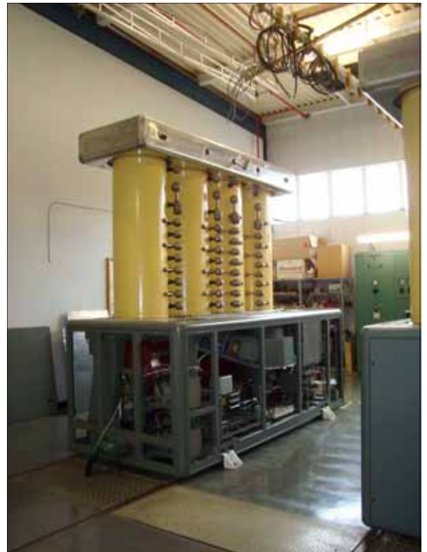
Mercury Arc Valve (HVDC) 1956
