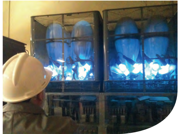
The glass-bulb mercury arc rectifiers of the Russell Place electricity zone substation.
