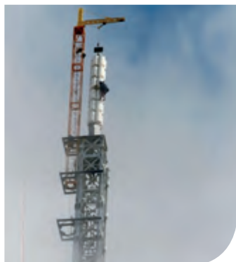
Working in the Clouds: Broadcasting Tower on Mt Wellington, Hobart, Tasmania. Photo taken by Tom Glass, Bruce Young Partners.
