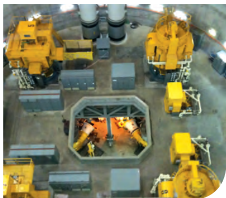
Hoppers Crossing Pumping Station – Site Tour.
