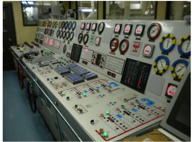
The Engine Room- Control desk
