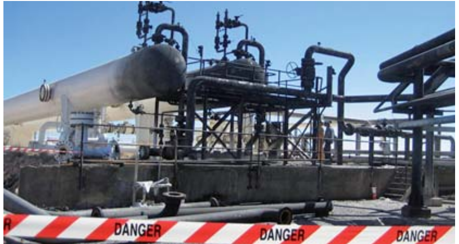
Fire damage at Apache Energy's Varanus Island facility.
