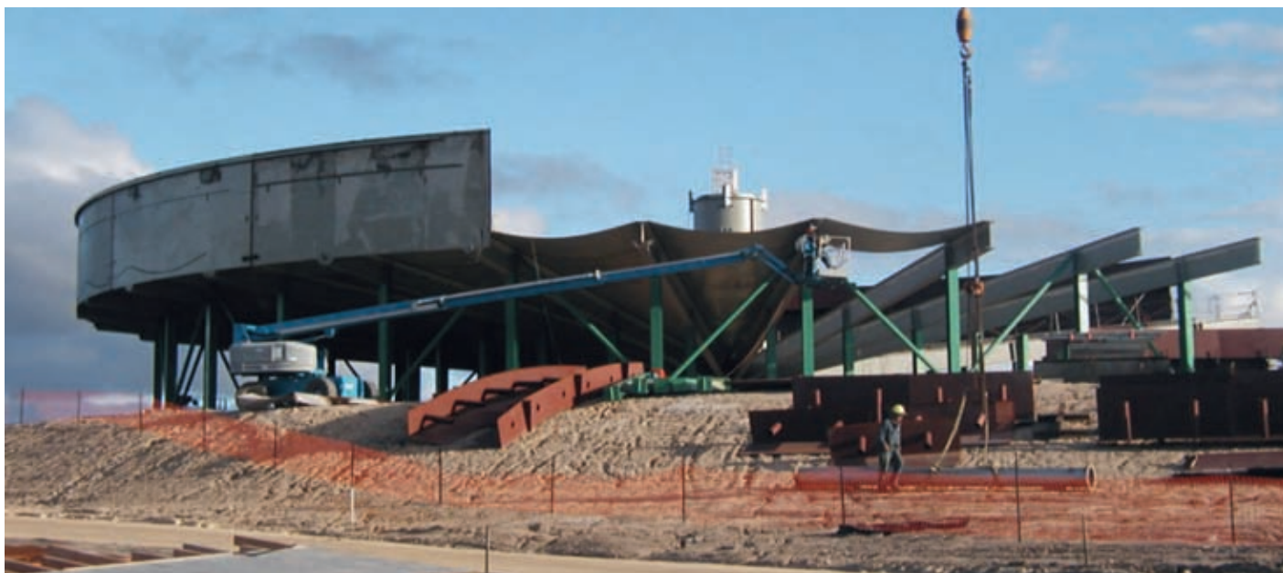
A picture of a similar thickener tank constructed at BHP Billiton's Mt Arthur coal mine in the Hunter Valley in NSW.
