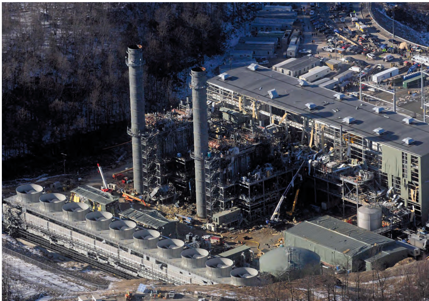
The Kleen Energy Systems powerplant in Middletown, Connecticut, US, shortly after the explosion.
