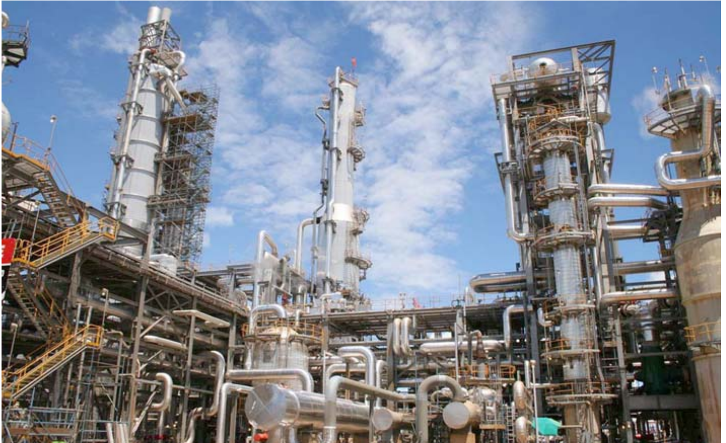
The new ammonia plant on the Burrup Peninsula
