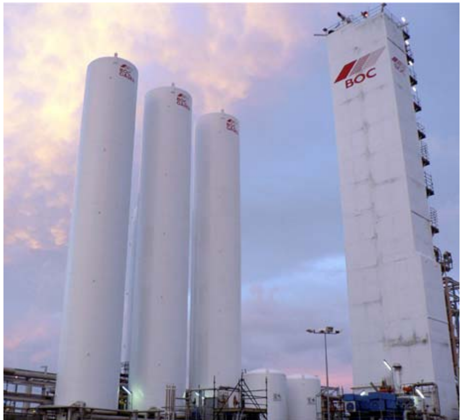
BP's Bulwer Island project near Brisbane has undergone an overhaul and upgrade. These gas separation units are part of the facility.
