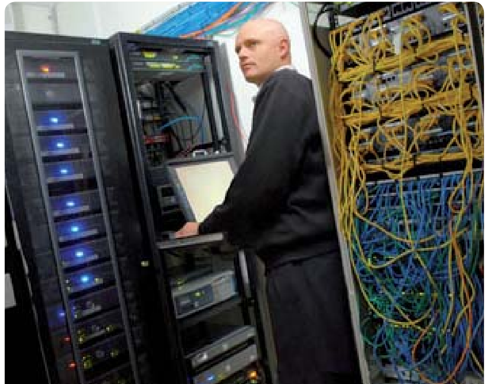
Andrew Dille, a member of the IT team, working in the network room of the company's head office in Warrnambool.
