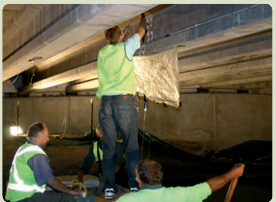
Fibre optic technology being installed underneath a bridge by the University of NSW's electrical engineering department for the Roads and Traffic Authority, NSW.
