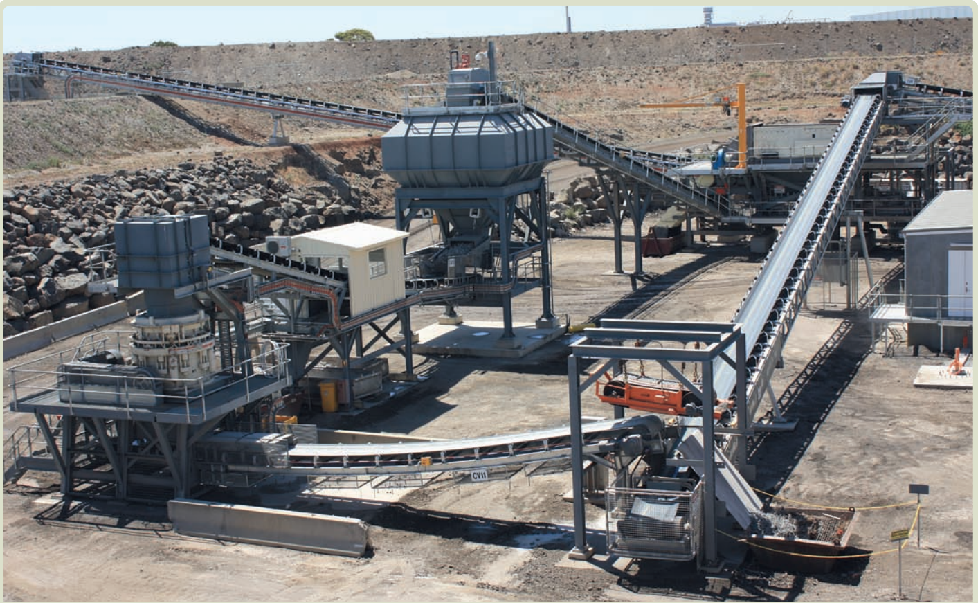
The completed recycling facility in Victoria, designed using computer aided design software.
