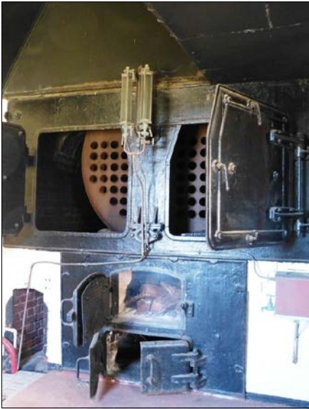
1916 under-fired, multi-tubed Trevor Boiler, which produced steam at 120 pounds per square inch until 1980 when the station closed. Ph: K.Baker.
