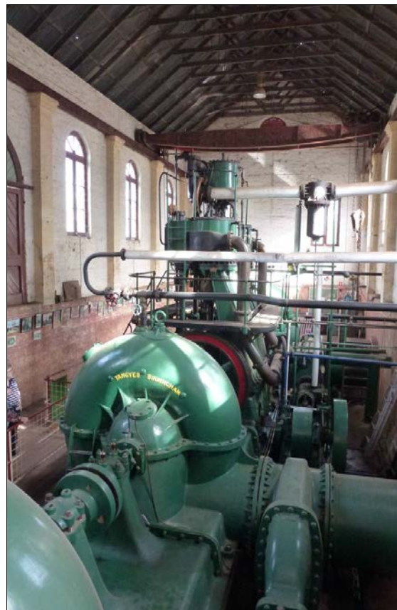
A view along the Psyche Bend Pumping Station with a pump in the foreground and the Tangye engine beyond.
