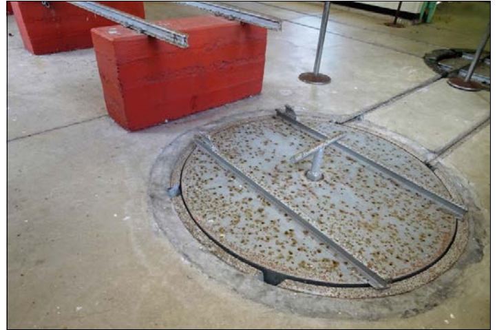
Elevating turntable to raise and turn incoming trolleys to the level of the rails into the steam chamber (see image at left). Photo: Keith Baker.
