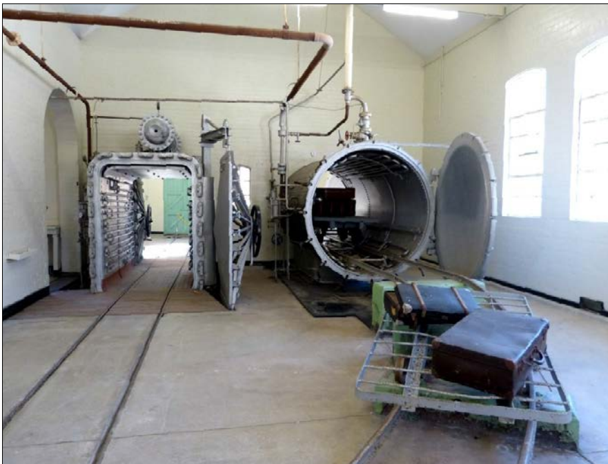
Trolley tracks emerging from the two disinfection chambers after treatment. On the right the trolleys return to floor level via a curved ramp. Note the colour of the rail support blocks changes from red (entrance side) to green (exit side) – ie. from foul to clean. Ph: K. Baker
