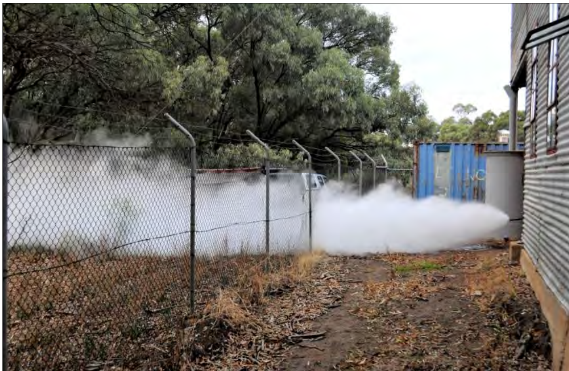
Blowing down the boiler to make sure the bottom spaces are clear of sludge (from the unpurified river water). Photo: Owen Peake.
