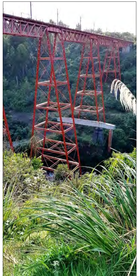
Image Right: The Makatote Viaduct, showing reinforcing of one tower foundation. Photo: Keith Baker.
