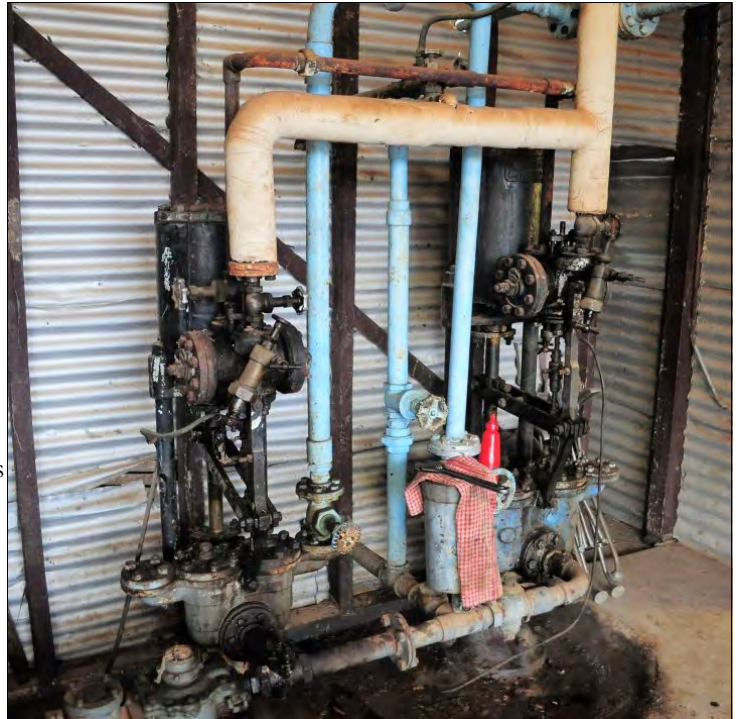
A bank of two Weir feed pumps, used to feed the Thompson boiler. The pumps take unpurified river water straight from the channel. On the day the author visited the site, only the right hand pump was operating. Photo: Owen Peake.
