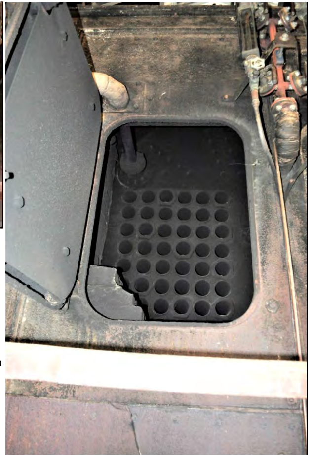
Fire tube nest with 42 tubes, behind the top left boiler door. The thin-walled fire tubes (but not the 10 thick-walled stay tubes) in each nest were replaced recently. Photo: Owen Peake.
