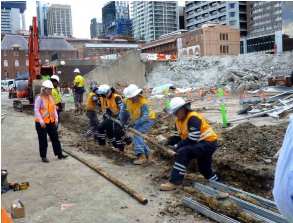
Left: The 2018 dig in William Street. Careful removal of full 20 feet lengths of Edison Street Tubes from the excavation. Photo: Brian Becconsall, February 2018.
