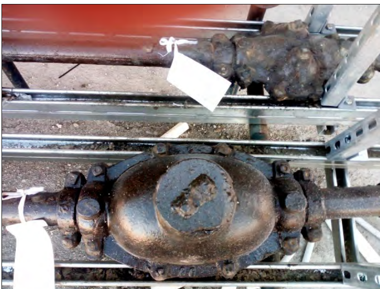
Below: Details of in-line joint “boxes” after preservation treatment. Photo: Brian Becconsall, February 2018.
