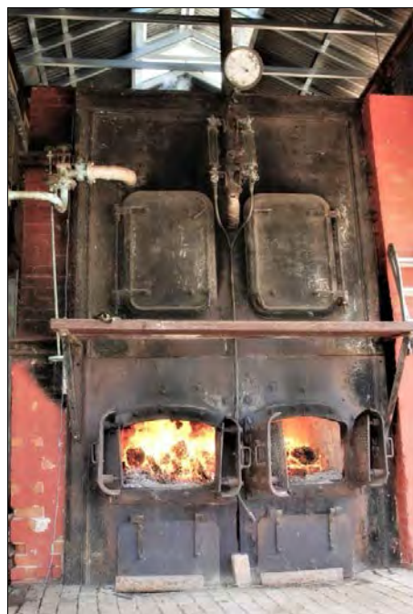
Image above: The front of the Thompson Colonial Boiler, with the two fire doors open. Photo: Miles Pierce.
