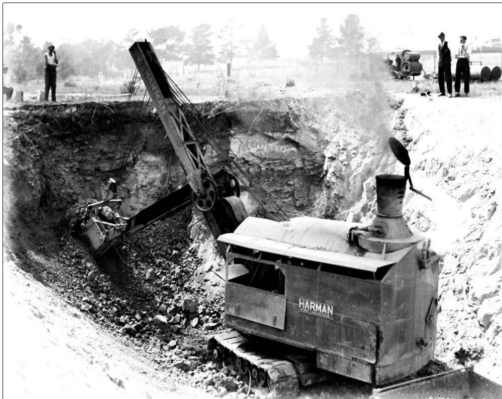
Harman steam shovel excavator used by Victorian Railways, c.1930. Source: Public Record Office, Victoria.
