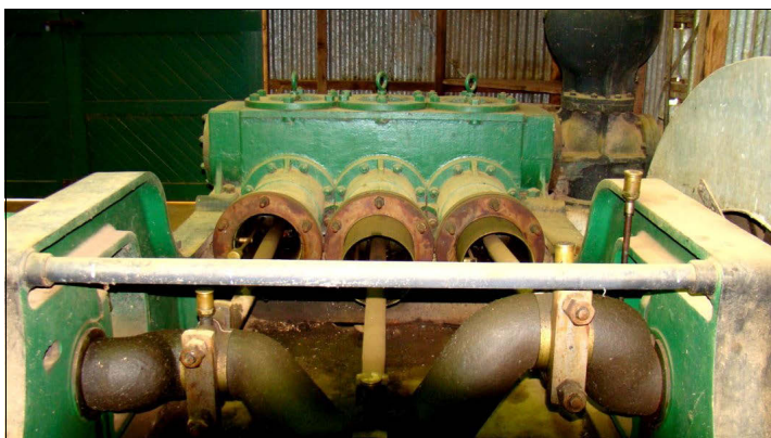
One of the triple ram piston pumps. Note the massive crankshaft and (at right) the curved safety guard over the speed reduction gear wheel.
