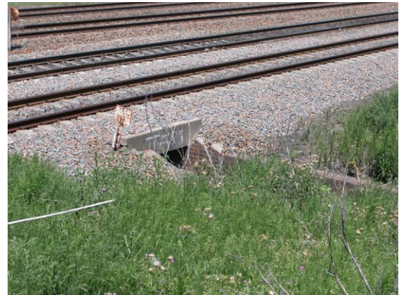
Photo 4: Original brickwork can be seen forming part of the culvert near Waratah—the brick channel beyond the culvert is of later construction.
