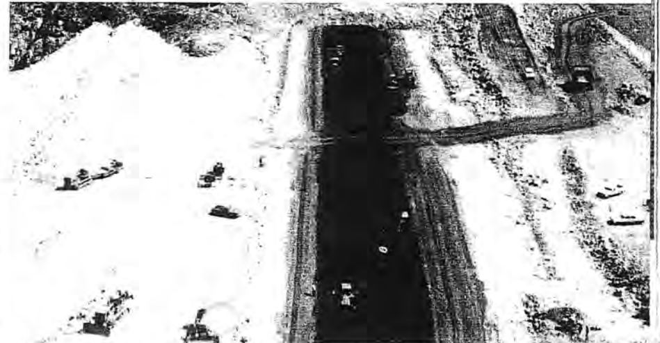
Partly completed embankment, August 1971. Rockfill zones are clearly shown on both sides of the central clay core
