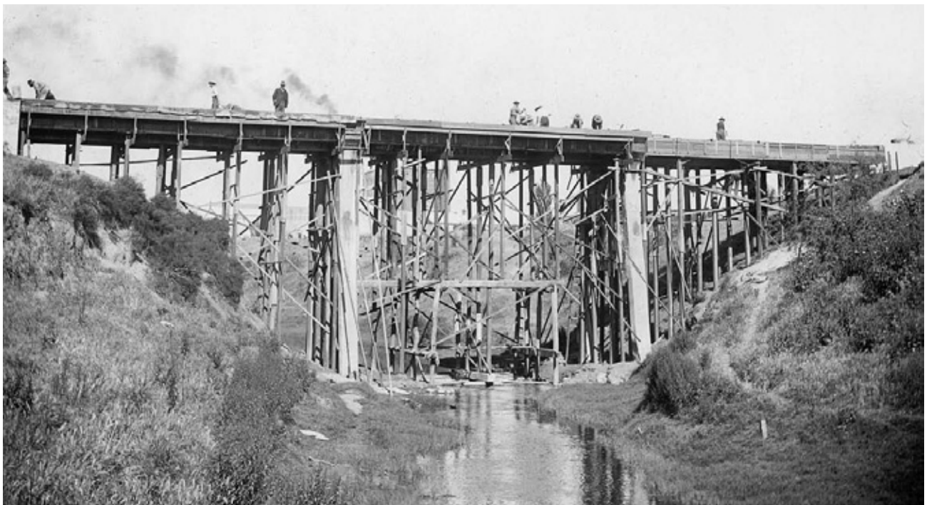
The Holland Street Bridge under construction – the trestles have been completed and concrete is being placed in the girder formwork (note man, right of centre, tipping wheelbarrow) [University of Melbourne Archives, BWP/24366 Reinforced Concrete & Monier Pipe Construction Co]
