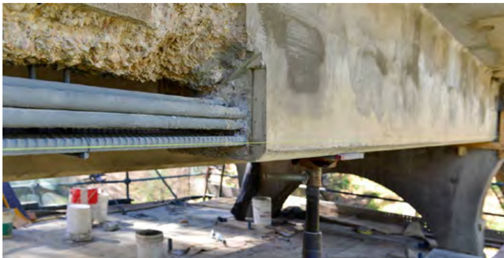
New concrete encloses the additional reinforcement and restores the bottom of the beam. This concrete has plasticisers with small aggregate and a strength of around 20 to 25 MPa to be consistent with existing concrete.
