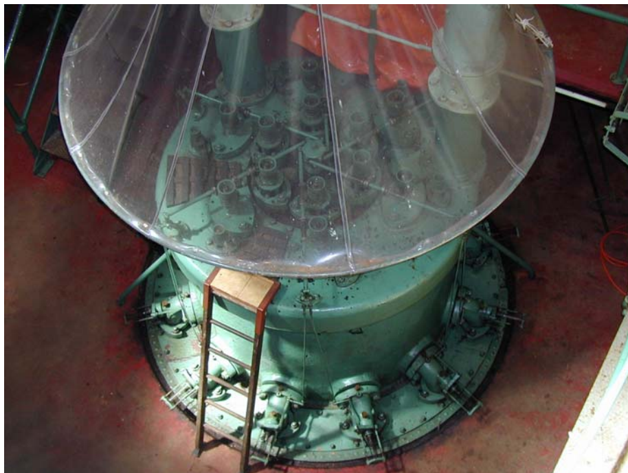
Photo 2: Top view of one of the pumps, taken from ground level. The green structure is the combustion head. The canopy above the pump is connected to a ventilating fan to remove any escaping gas.
