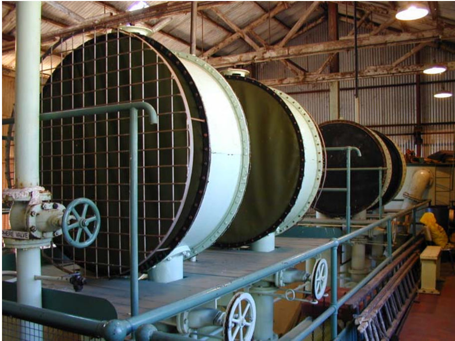
Photo 3: the gas bags with the gas supply pipe and valves at the front. The gas pipes to the pump can be seen at the rear of the distant bag.
