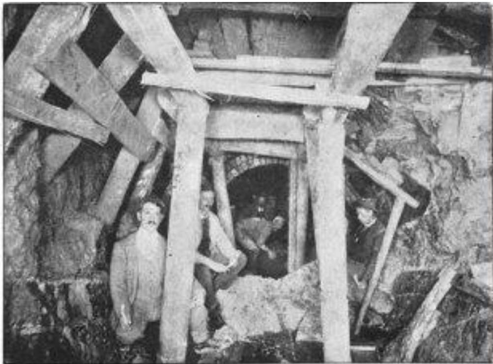
Plate XLV.—No. 6 Section, North Yarra Main Sewer, showing timbering in excavation for brick work and brick lining in background.
