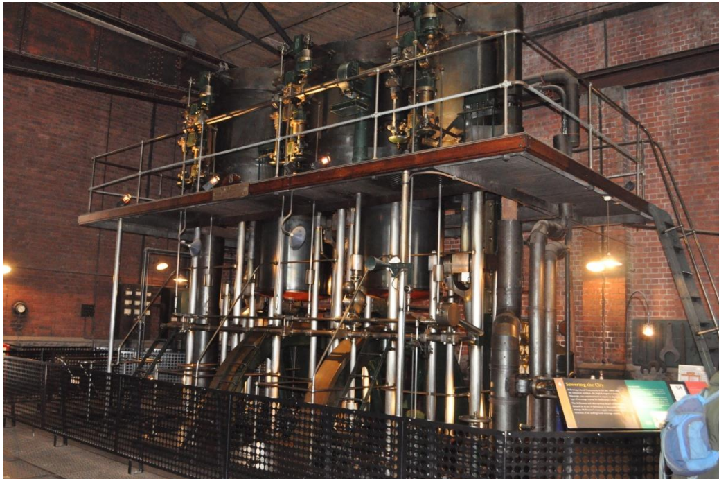
Austral Otis pumping engine No.8 at Spotswood. Image: Owen Peake
