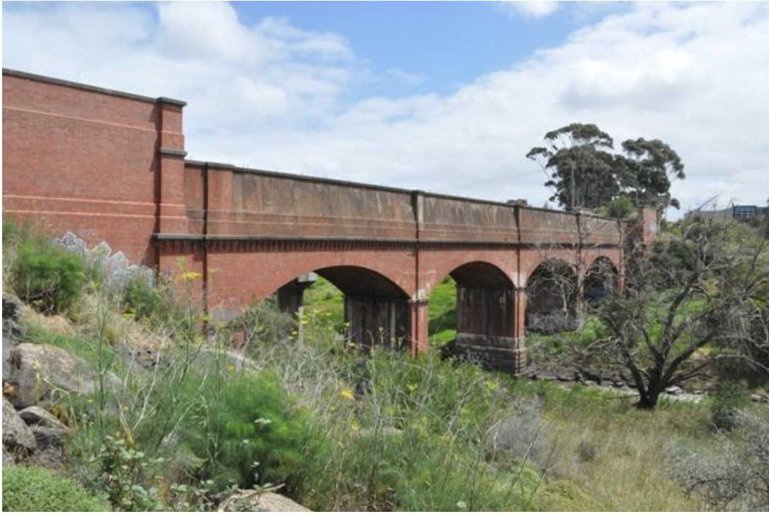
Kororoit Creek aqueduct on the original Main Outfall Sewer. This sewer is now out of service and the aqueduct has been converted to a cycle path. Image: Owen Peake
