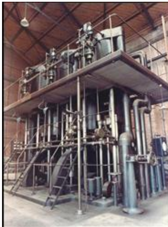
No.8 Austral Otis Pumping Engine, Spotswood Pumping Station, 1982
