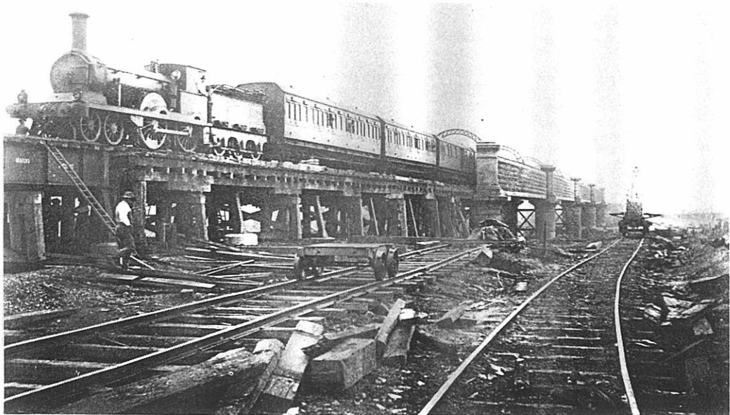
Dubs D class loco with up Melbourne express crossing last of the timber girders onto a steel girder which has just been place.
