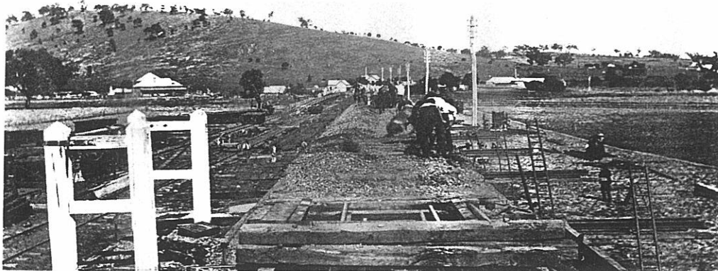
Rails and sleepers removed from the length of deck to be demolished. Deck has also been jacked up to permit placing of slide rails between corbels and headstocks over each timber pier.
