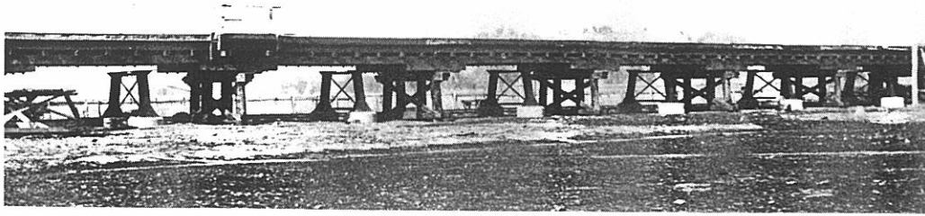
The first stage - steel piers constructed on concrete footings under existing timber girders.
