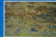
Northern side of southern arch, re-pointing, mortar loss and leaching prior to restoration in 2000
