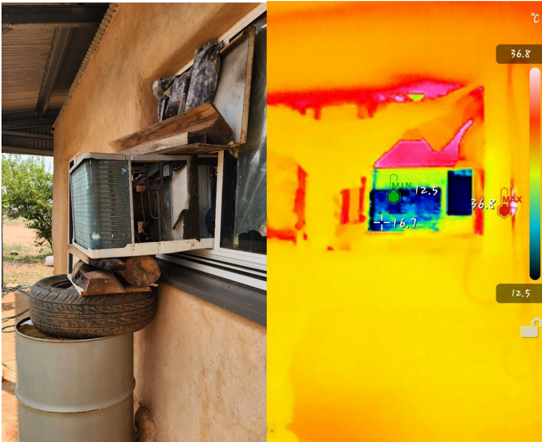
Box AC in window with infrared image showing heat coming into the house around it
