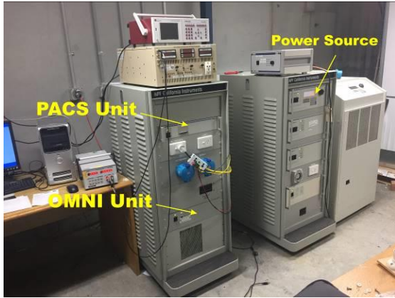
Fig. 1. Large 3 phase H&F Test System.
