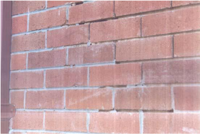
Mortar Weakened Wall
