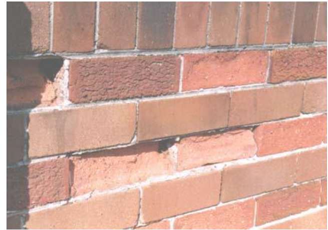
Salt Attack in Clay Bricks
