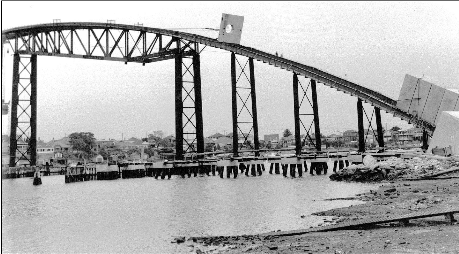
Precast diaphragm unit making its way along falsework track by trolley and winch
