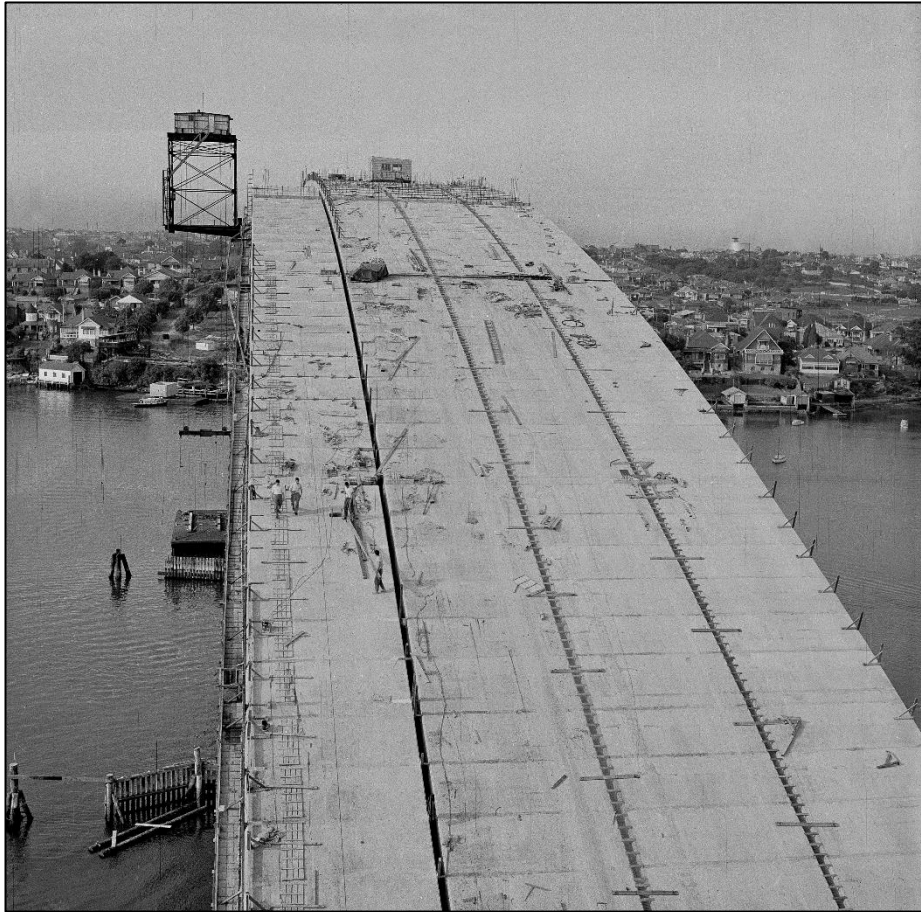
Note 230mm (9 inches) gaps between arch ribs (subsequently used for post-tensioning tendons)
