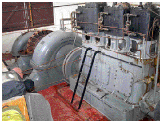
Millewa 'A' Pumping Station Thompson engine and Weymouth centrifugal pumps
