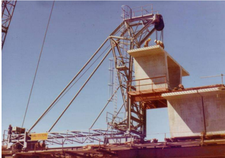
Figure 11. Unit transporter connected to placing gantry prior to lifting (Photo J O Clough & Son)
