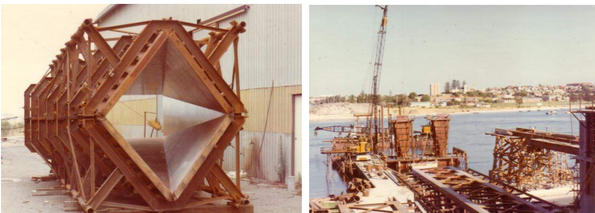
Figure 8. Left: Steel pier column forms; Right: Placing the forms on the pile cap (Photos J O Clough & Son)
