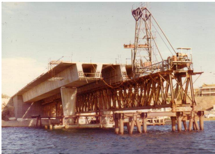
Figure 12. Stage 1 upstream row completed, downstream row placed but not yet stressed. (Photos J O Clough & Son)
