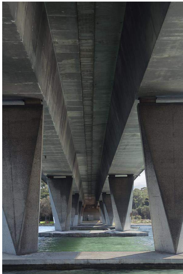
Figure 5. View of the underside of Stirling Bridge looking north. The view highlights the clean lines of the bridge beams and the architectural profile of the columns (Photo Anthony Riddette)
