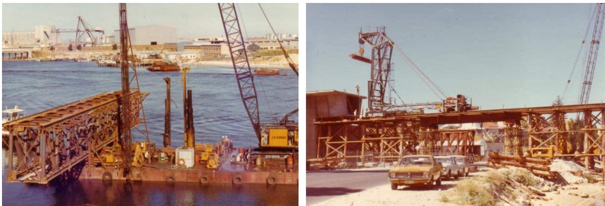
Figure 10. Left: Truss section being moved into place by crane barge; Right: South shore span falsework with placing gantry in position (Photos J O Clough & Son)
