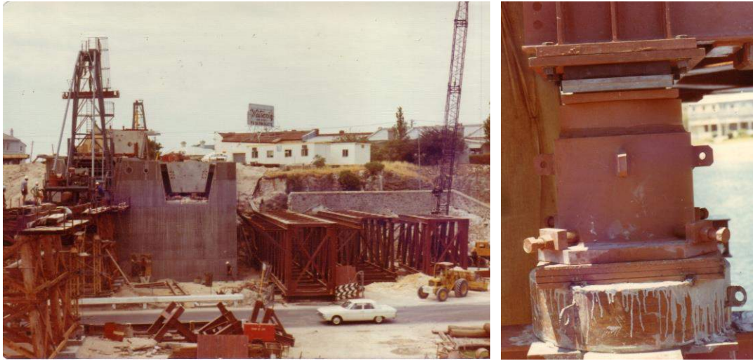
Figure 9. Left: Assembly of falsework trusses on south bank; Right: 200t capacity sand jack (Photos J O Clough & Son)
